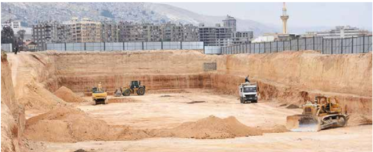
Construction work at the site of Marota City project. One of the projects of Cham Holding. The land of the project was previously occupied by informal houses. Source: Marota City website.
