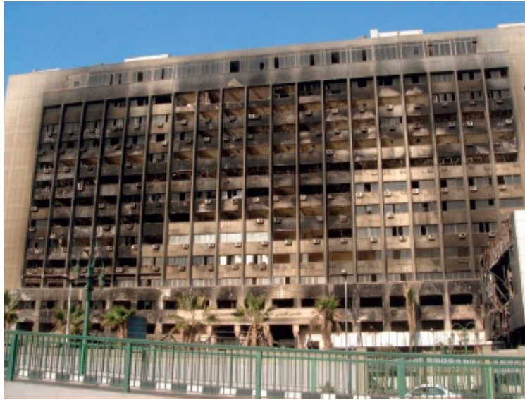
Mubarak's National Democratic Party headquarters in Tahrir Square gutted by fire
